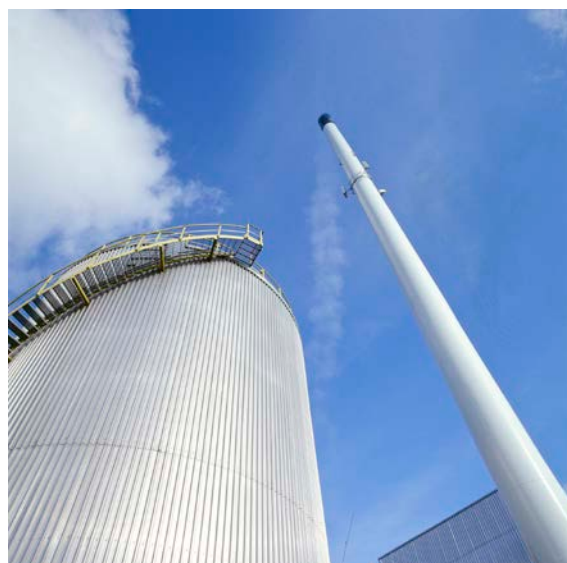
Incineration plant, Denmark
